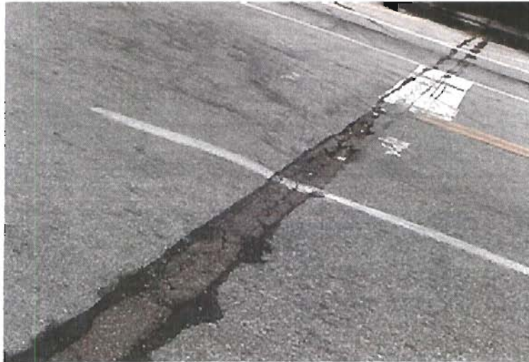
EX. JOINT UNEVEN
