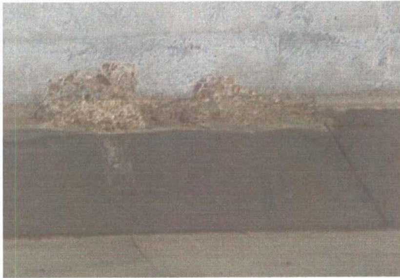
BEAM A, SPAN 2, LARGE SPALL
