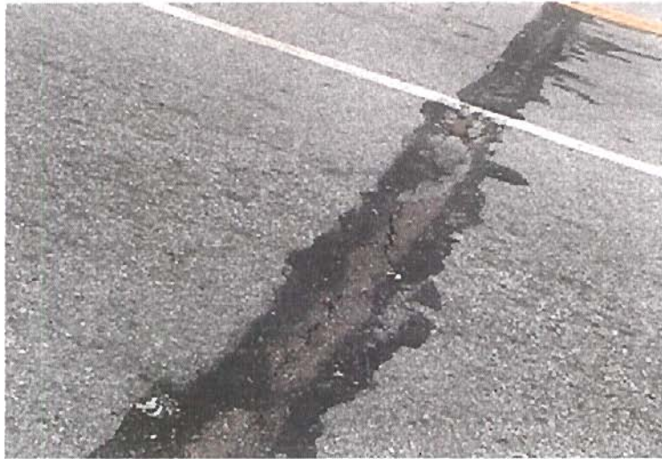
EX. JOINT UNEVEN
