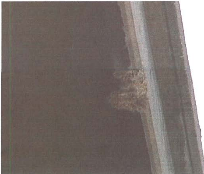
SPAN 3, BEAM A, SPALL
