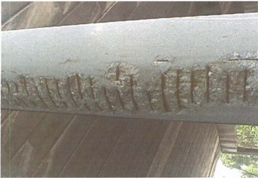
BENT 3, COLUMN A, REBAR SPALL, REINFORCING EXPOSED
