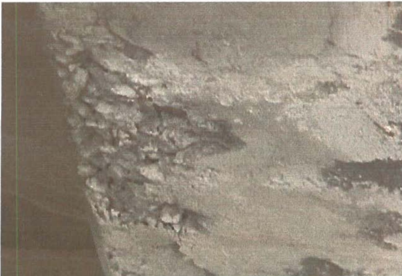
BENT 1, LARGE SPALL WITH HONEYCOMB AREAS
