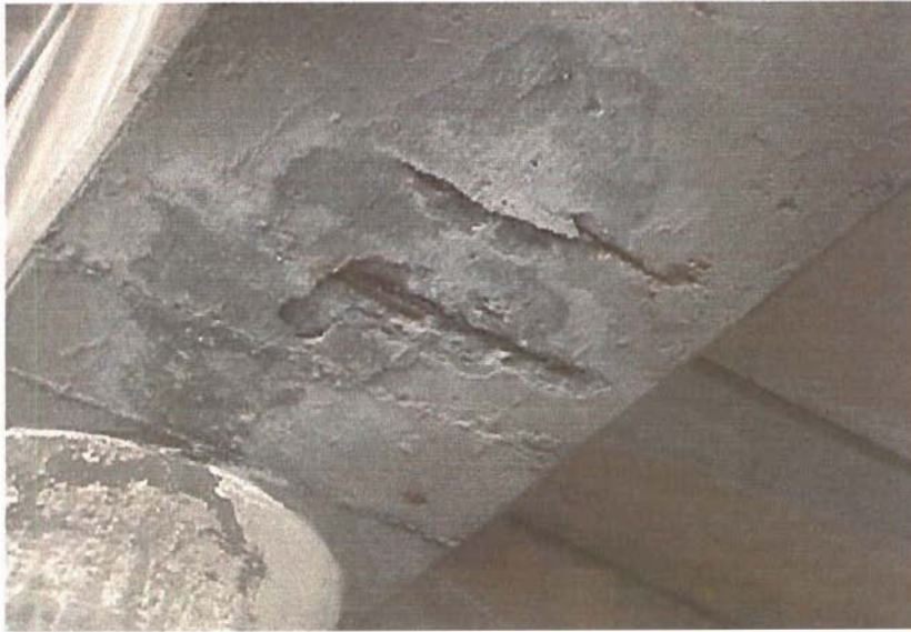
BENT 1, LARGE SPALL WITH REBAR EXPOSED
