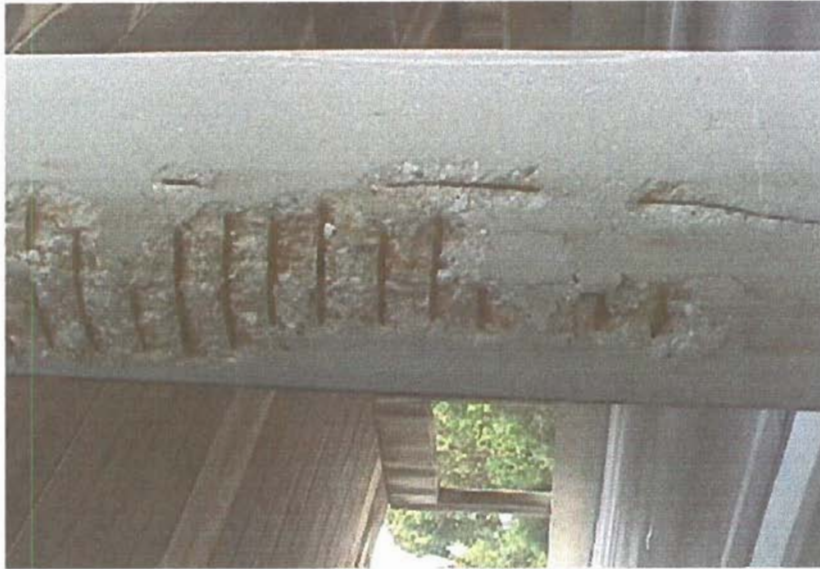
BENT 3, COLUMN A, REBAR SPALL, REINFORCING EXPOSED
